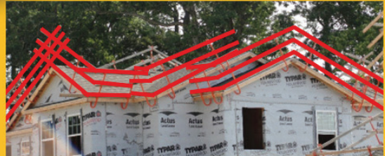
Proper fall protection: Roofing job surrounded by horizontal under-eave guardrail system, a “safety by design” structure that protects against falls from any location on the worksite.
